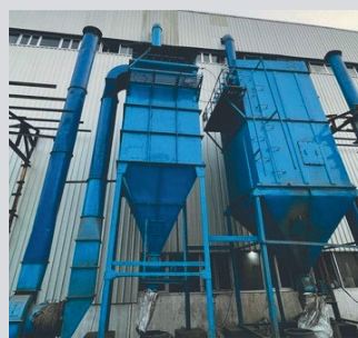
DUST COLLECTOR PLANT
